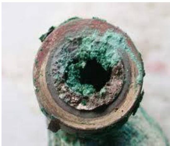
Pipe Corrosion Inside Plumbing
