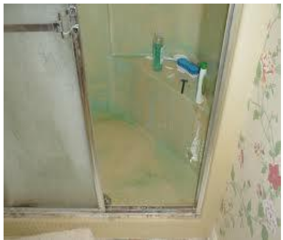
Visible Effects of Pipe Corrosion
